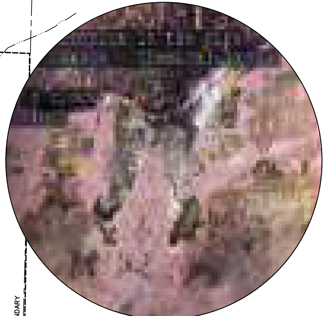
SEVERE MATERIAL DAMAGE (MANHOLES 35-34)
